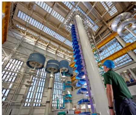
High voltage test lab at the power transformer factory in Stafford, United Kingdom
