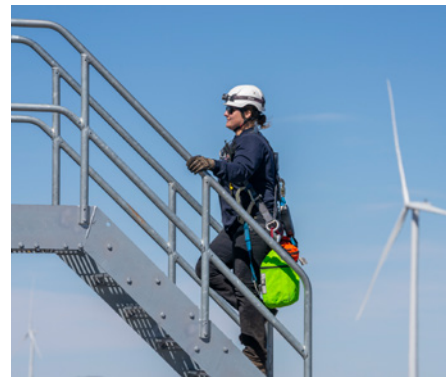
A technician performs maintenance on a GE Vernova onshore wind turbine in New Mexico
