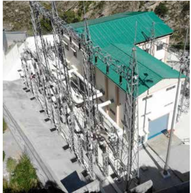
66 kV Gas Insulated Substation for HPPTCL at Urni
