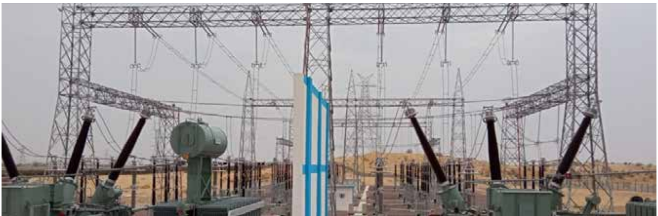
Three 132 kV Air Insulated Switchyard (AIS) bays commissioned for Sterlite in North Eastern Region Substation package at Surajmani Nagar
