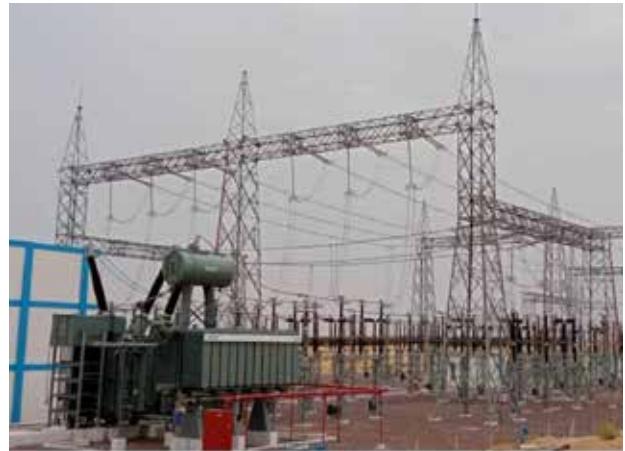
Energized 400kV GSS, RSS with 150MVA Trafo & 12x12.5 MW ICRs for Azure Power at Bikaner
