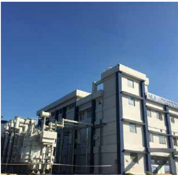
220 kV Gas Insulated Substation (GIS) bays and 160 MVA Transformer commissioned for Kerala State Electricity Board (KSEB) at Kaloor
