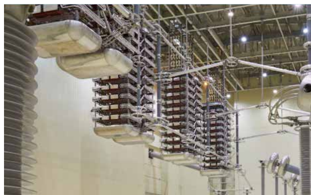
Commissioned Pole-4 of Champa Kurukshetra Phase-2 project for PGCIL. With commissioning of the fourth pole, the capacity of Champa-Kurukshetra transmission link has increased to 6000 MW
