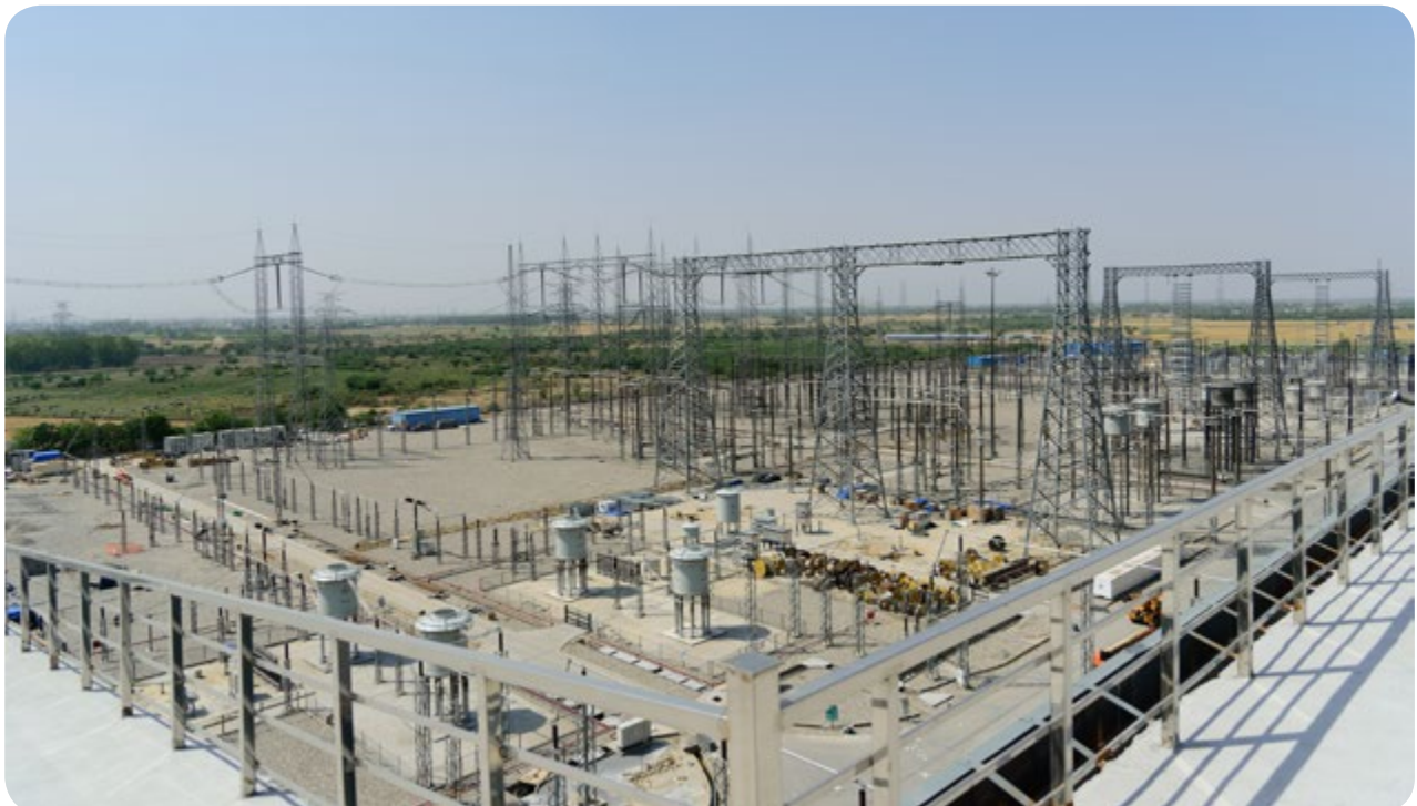
▲ HVDC site for Power Grid Corporation at Kurukshetra, Haryana
