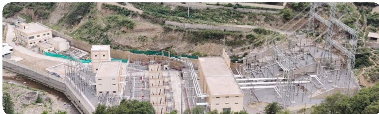
400 / 220 kV GIS Sub Station at Gumma, Himachal Pradesh
