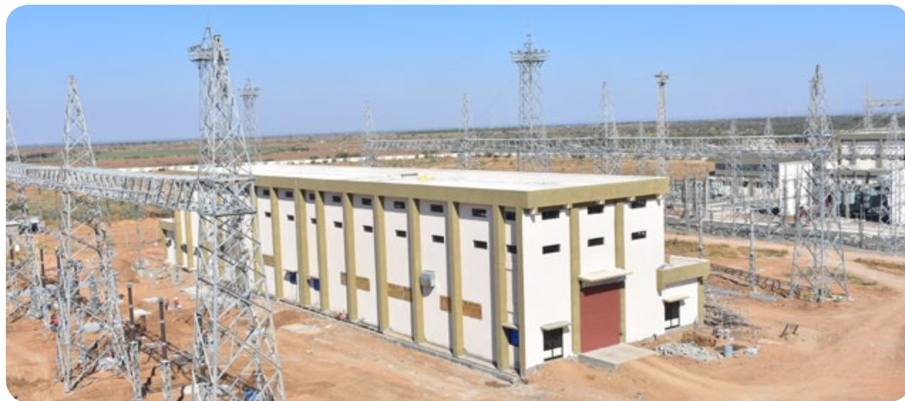
400 kV Gas Insulated Substation for Gujarat Energy Transmission Corporation Limited (GETCO) at Bhachunda, Gujarat
