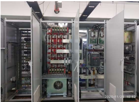
Excitation system upgrade NHPC Chamera-II (3X100MW)
