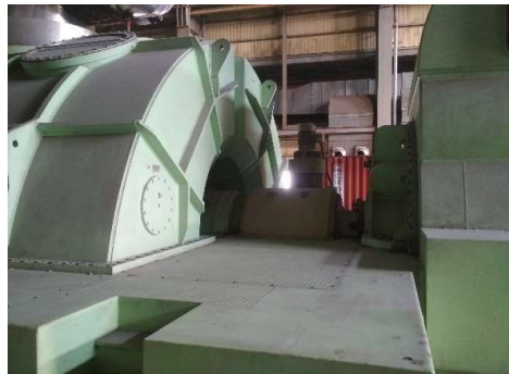
Resolving fly ash erosion problem Unit#2 Adani Chinese OEM
