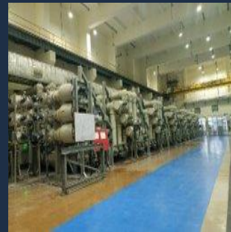
HMEL, Bhatinda, Punjab Commissioning of 400kv 12 GIS bays along with 250MVA 2 nos. transformers
