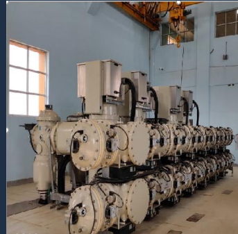
WBSETCL Manbazar Full Commissioning of 132kv 6 GIS bays , 33kv 15 GIS bays and 2x31.5MVA transformer Substation
