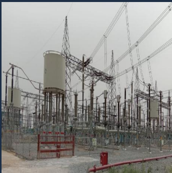
Adani , Mohindergarh, Haryana Commissioning of Dhanoda Line 1 GIS bay & line 2 AIS bay for 400kv Series Reactor
