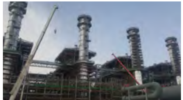
1270 MW Wad al Shamaal (with Solar field) CCGP - Power Block
