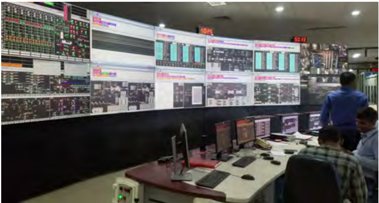
2X660MW Solapur Thermal Power Plant Unit#1 CCR
