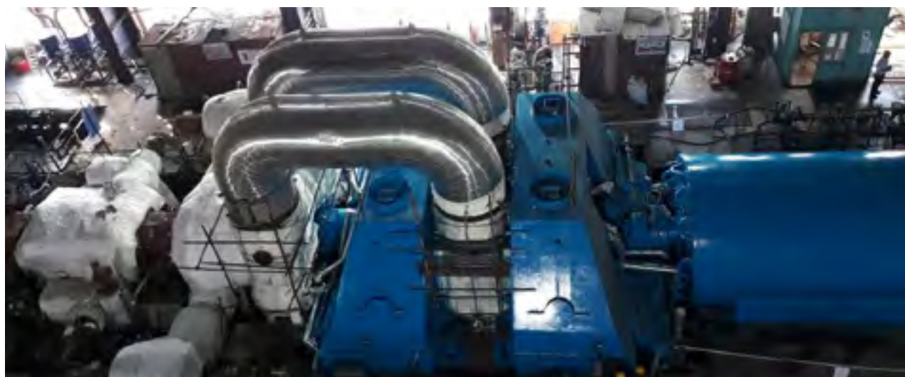
Ukai Thermal Power Plant
