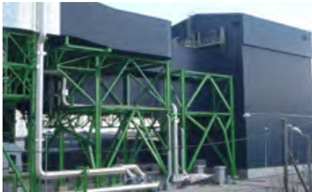
1X150 MW Sihanoukville, Cambodia Power Plant
