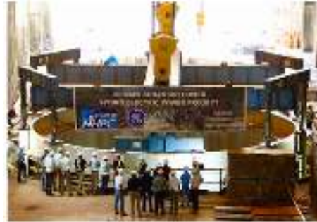
Stator assembly for unit 1 into the generator pit Subansiri lower hydro electric power project
