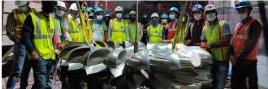
Erected the Runner of Unit 1 & lowered the stator and rotor for Unit 2 Tidong project
