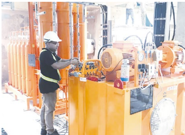
Commissioning Engineer working on Governing System Oil Sump tank at Da Nhim Hydro Project site in Vietnam
