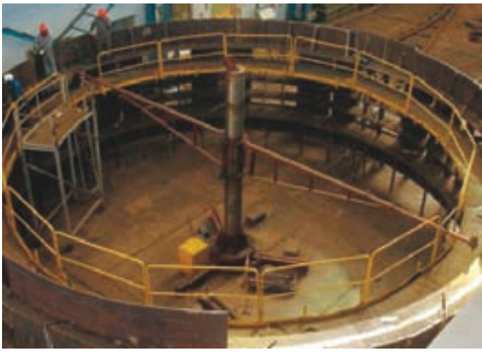
Subsiri 8 x 25 MW - Stator Frame Fabrication of 14 Meter Diameter at Vadodara Workshop
