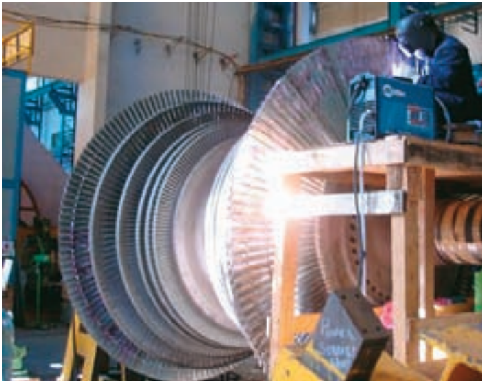
NLC LP Rotor Lacing Wire Bridge Welding at Power Service Workshop at Vadodara
