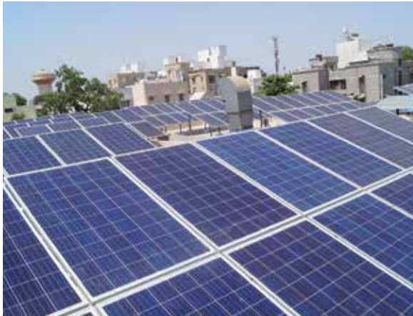
Solar panels erected on the roof top of Akshaya Patra Foundation's Kitchen, Vadodara
