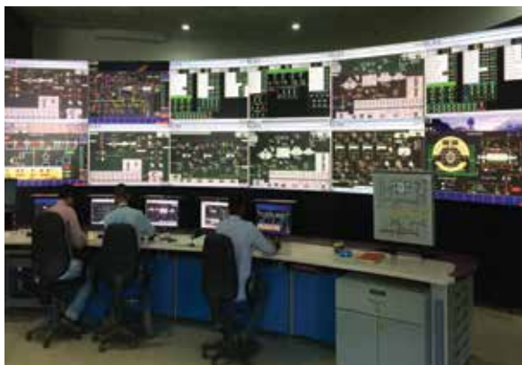
Control Room at NTPC Mouda II 2x660MW, Steam Thermal Power Plant
