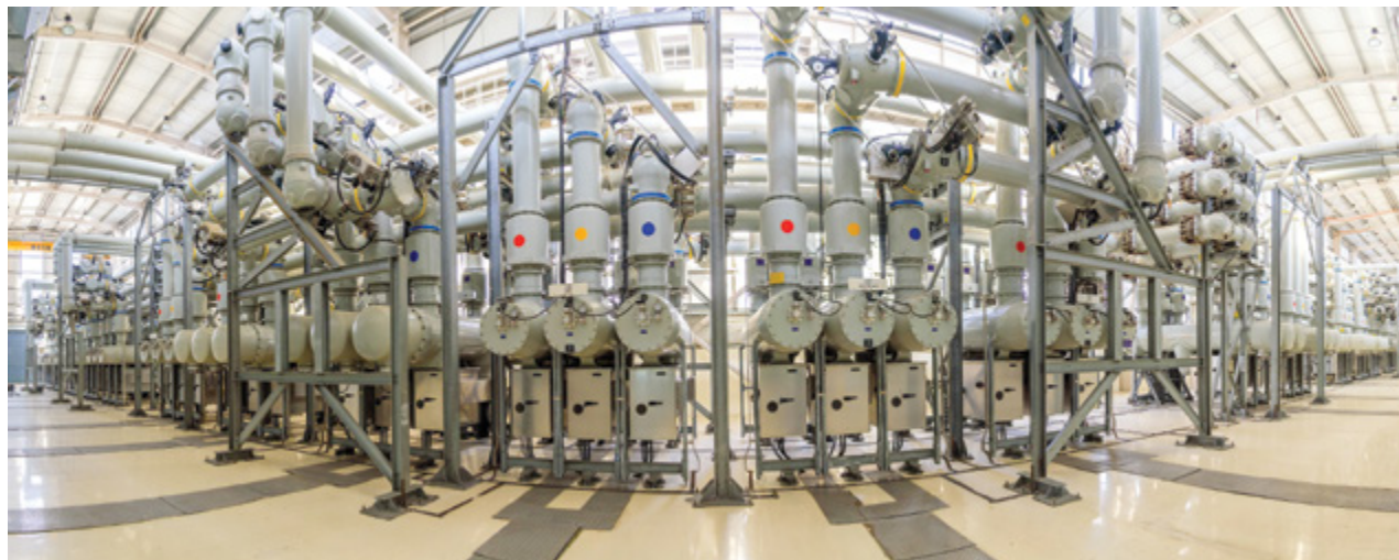
765kV GIS HVDC site, Kurukshetra
