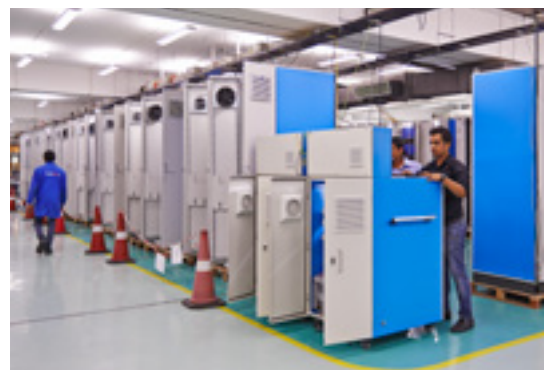
Automation & Control office in Noida
