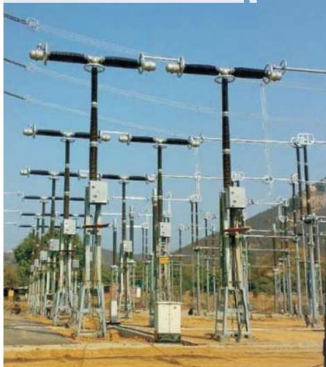
765 kV GL318D commissioned at Unit II of Lanco's Anpara - C Project in Sonbhadra (Uttar Pradesh).
