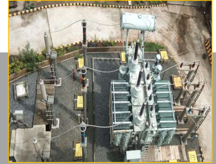
Energized 132kV 40 MVA 2 nd trafo issued by OPTCL at Bhubaneswar
