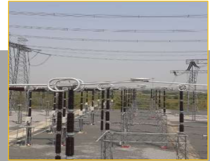
Energized 765kV 1 AIS bay for GTL ADANI Extn package at Gr. Noida
