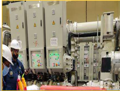
Commissioned 132 kV 40 bays of GIS for HMEI at Bhatindra
