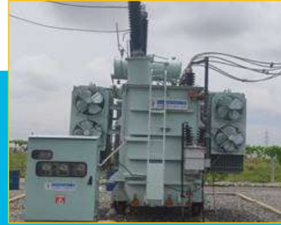
Commissioned 132 kV 2 bays for OPTCL VO of GIS Extn at Chandbali
