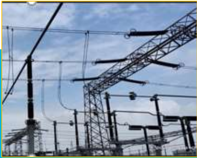
Energized 765kV 2 bays of Generator Trafo#2 with Tie Bay for NTPC, Darlipalli
