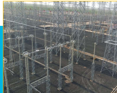
Commissioned 400 kV 03 bays & 220 kV 06 AIS bays for PGCIL at Bhuj
