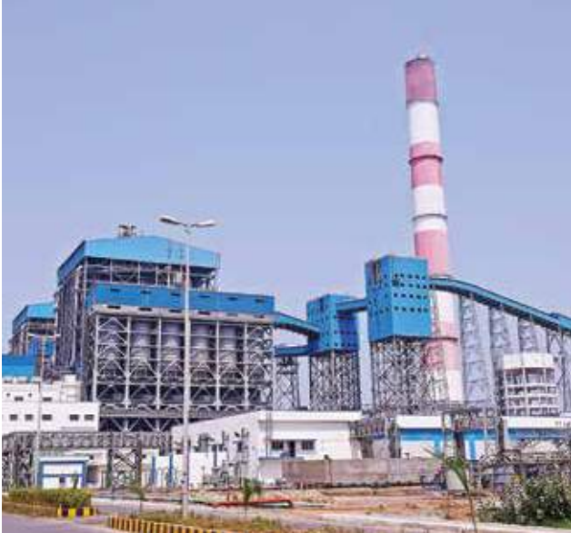
First unit of Krishnapatnam Supercritical Thermal Power Plant (2x800 MW) at Andhra Pradesh starts commercial operations
