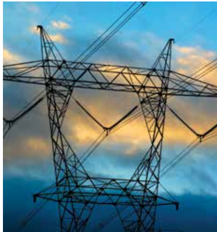
> Transformation of existing grid infrastructures
