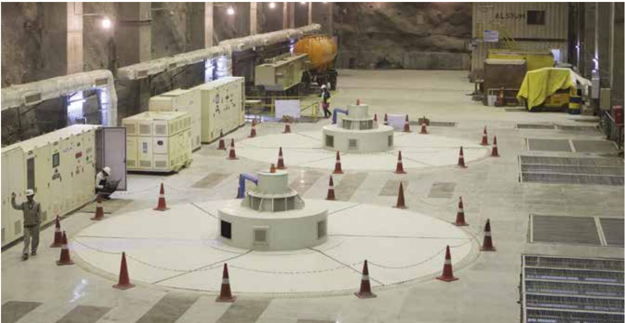
3x77MW Chamera III hydropower project in Himachal Pradesh
