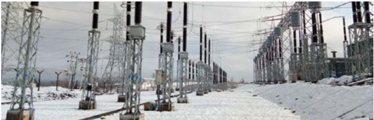
400/200 kV Gas Insulated Substation situated at an altitude of 2024 mts (6640 ft) in the Amargarh village of Kashmir
