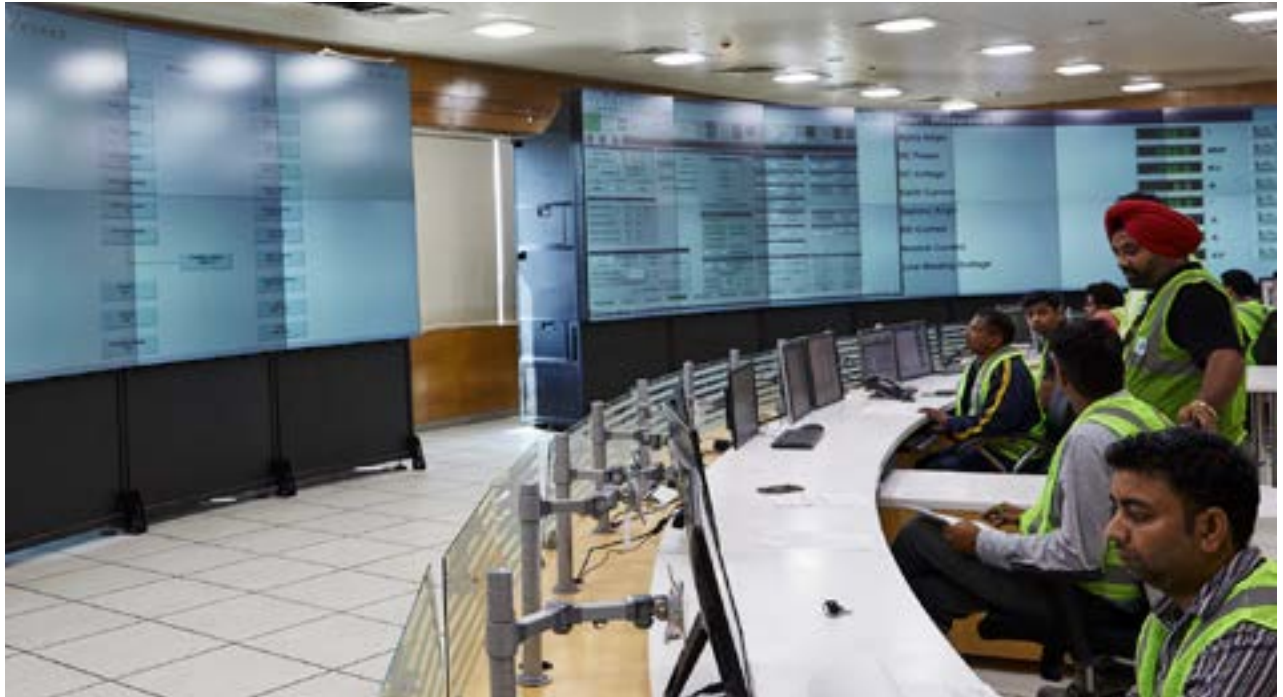
Champa Kurukshetra Project : Control Center at Kurukshetra
