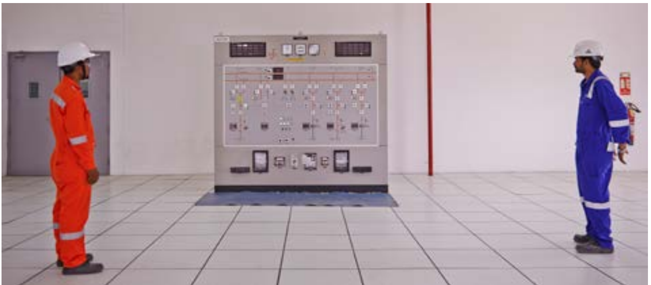
Grid Automation Unit - Pallavaram
