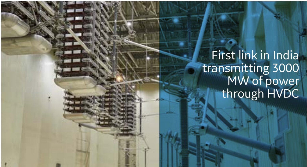
Valve Hall 765 kV HVDC at Kurukshetra
