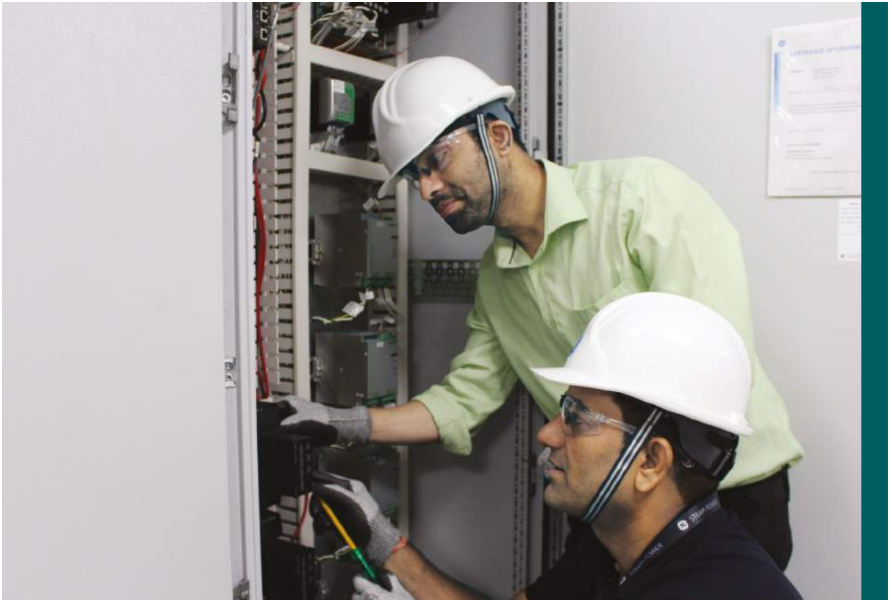
Employees at work at the Automation and Controls facility in Noida
