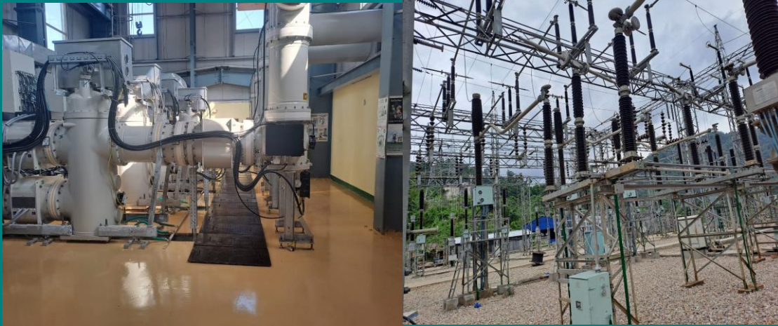
132KV GIS bays at Powergrid Kopili
