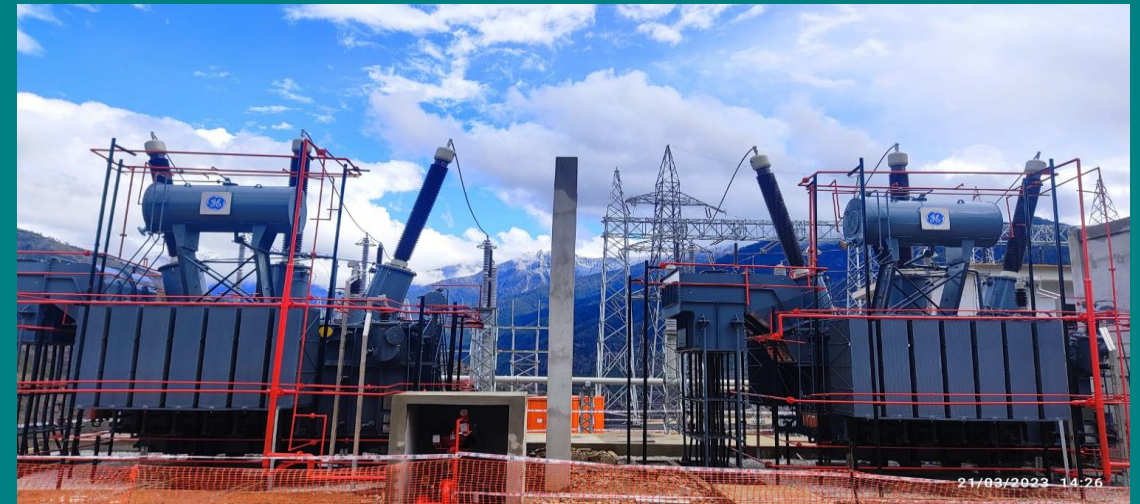
220/66 KV GIS bays– 80MVA trafo commissioning at BPC Chumdo
