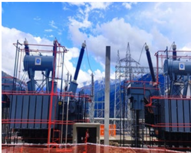
GE's first 220 kV Gas Insulated Substation in Bhutan for Bhutan Power Corporation
