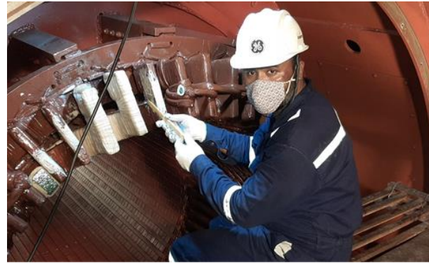
Local repair followed by all required testing of Stator/Rotor for Jaypee Bina thermal power plant
