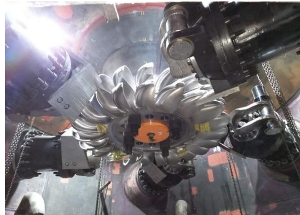
Turbine and generator rotor shaft of Unit 1 was rotated for the first time for Tidong project
