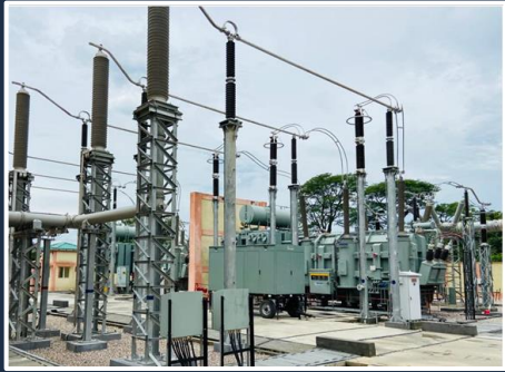
1 X 100 MVA ICT Commissioned at HPPTCL Dehan, HP
