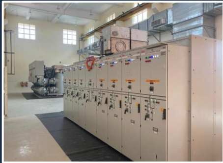
1 X 20 MVA, 132/33 kV Transformer along with 5 bays of 132 kV GIS and 9 bays of 33 kV GIS commissioned at OPTCL Hinjilicut, Odisha
