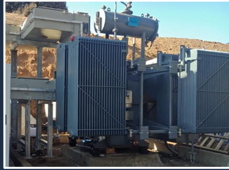
4 X 5 MVA, 33/ 0.415 kV Transformer Commissioned at BPC Samcholing, Bhutan
