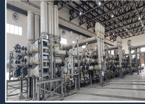
3 X 400 kV GIS bays at Doosan Jawaharpur out of 15 X 400 kV GIS Bays in UP
