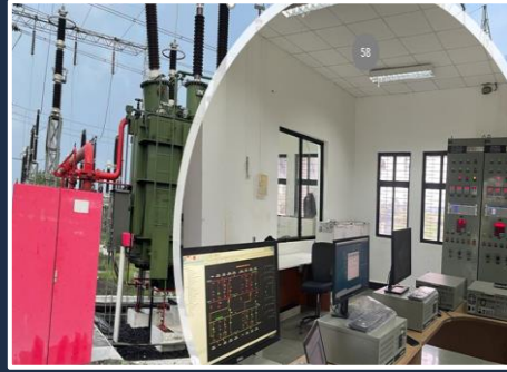
2 X 100 MVA ICT Commissioned at Pimpalgaon Substation, Maharashtra
