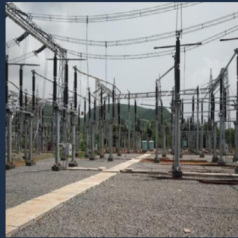
5 bays 220kV GIS Substation along with line 220 kV 1&2 with associated 220kV AIS Outdoor equipment's, Bus 1&2 & Buscoupler for HPCL at Vizag
