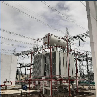
400kV Bus Reactor for PGCIL at Thiruvallam
