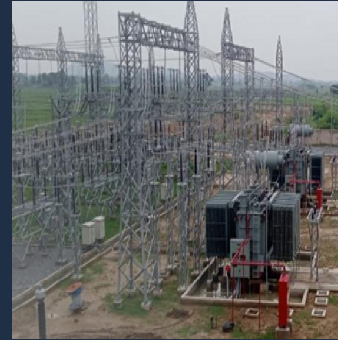
2 X 50 MVA, 132/33kV along with 9 X 33kV Bays at JUSNL at Naudiha
