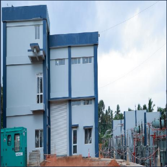
220/110kV 06 GIS Bays for KSEB at Vizhinjam
