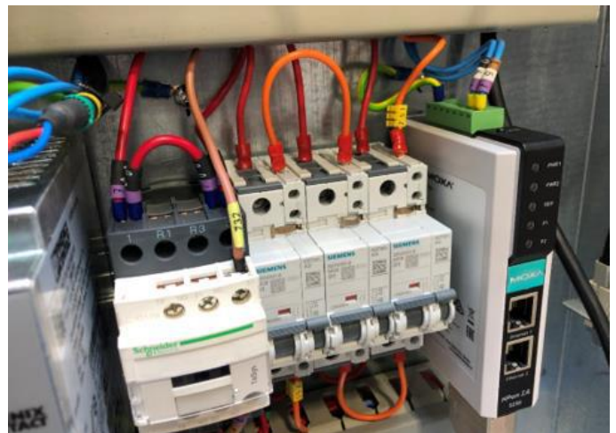
Cooling Kit MCB's installed and wired ready for test
