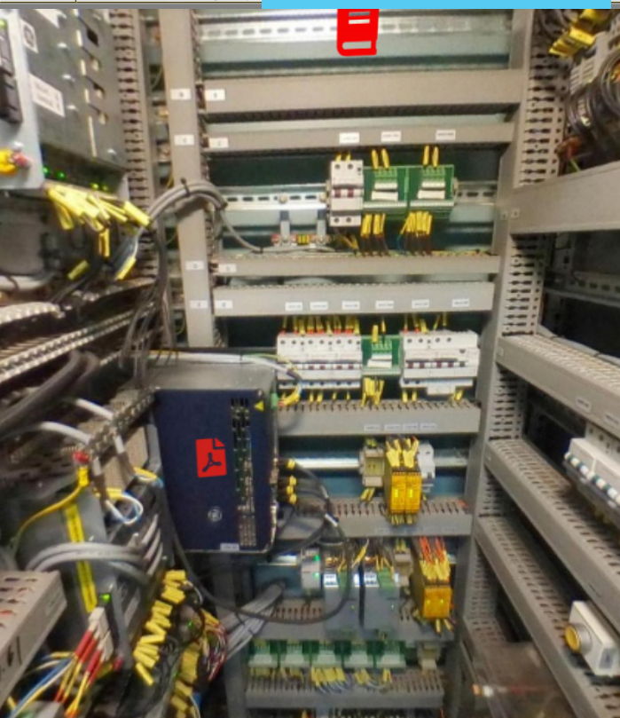
Control cubicle 360° view
