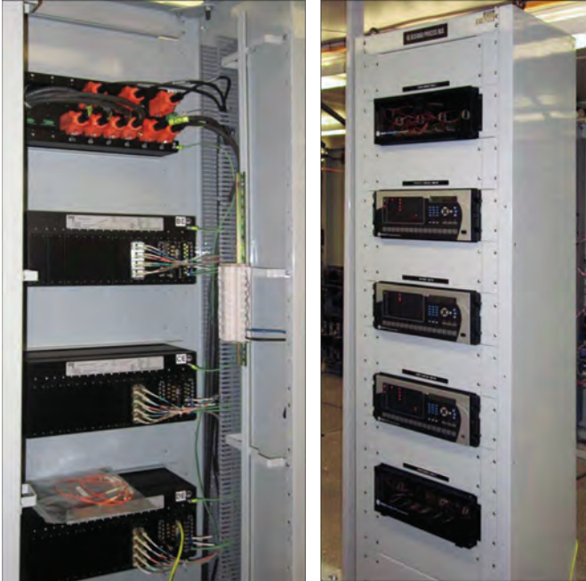
Figure 2. HardFiber protection panel with three relays and two patch panels (top and bottom). All I/O signals interfaced via fiber optic communications.
