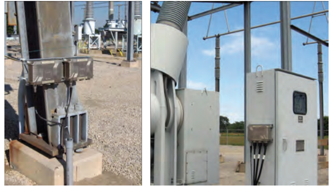
Figure 4. HardFiber bricks installed on a bus support structure (left) and a breaker marshaling box (right).
