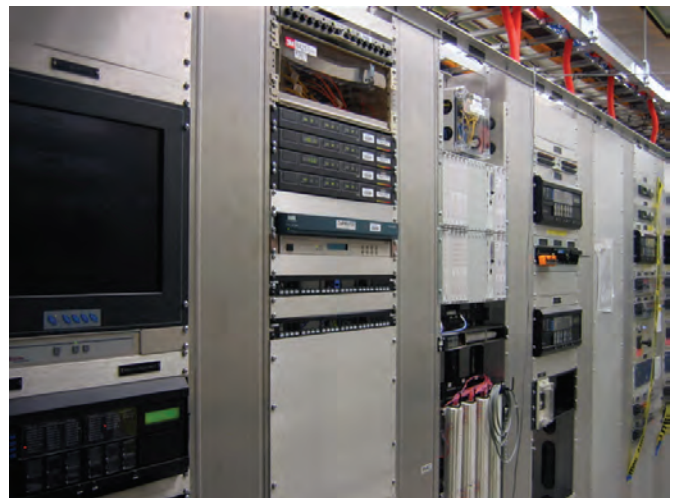
Figure 14. Typical MPAC Building Showing the HMI
