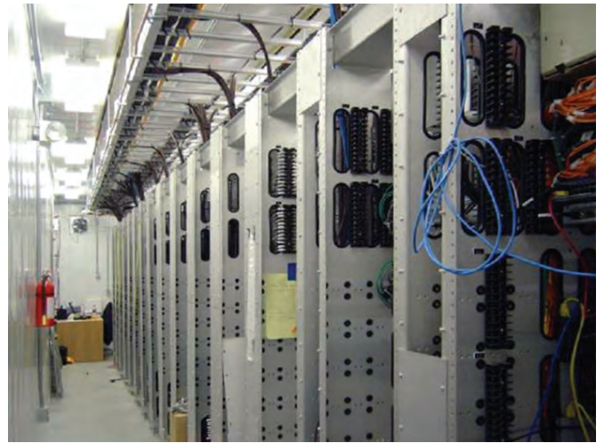
Figure 13. MPAC Building – Minimized Wiring
