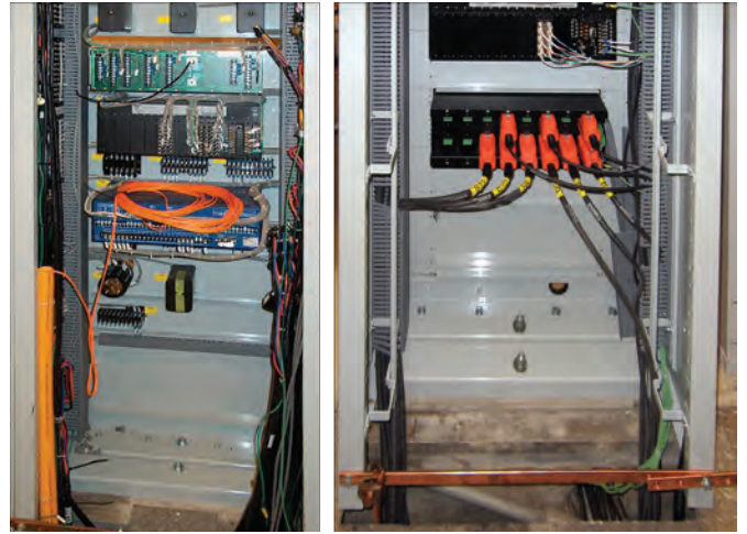
Figure 6. Before (left) and after (right) — the amount of cabling at relay panels is greatly reduced.
