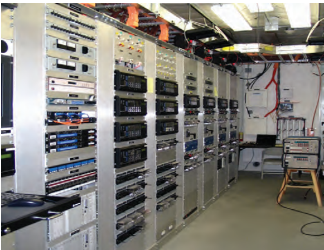
Figure 12. MPAC Building with Integrated Protection and Control
