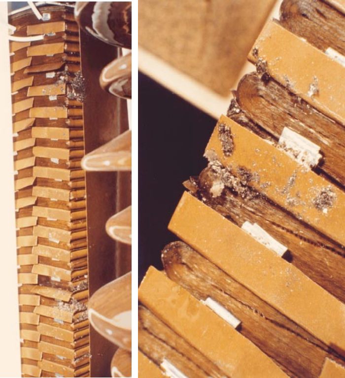
Fig. 5. Examples of failed CCVT capacitor stacks.
