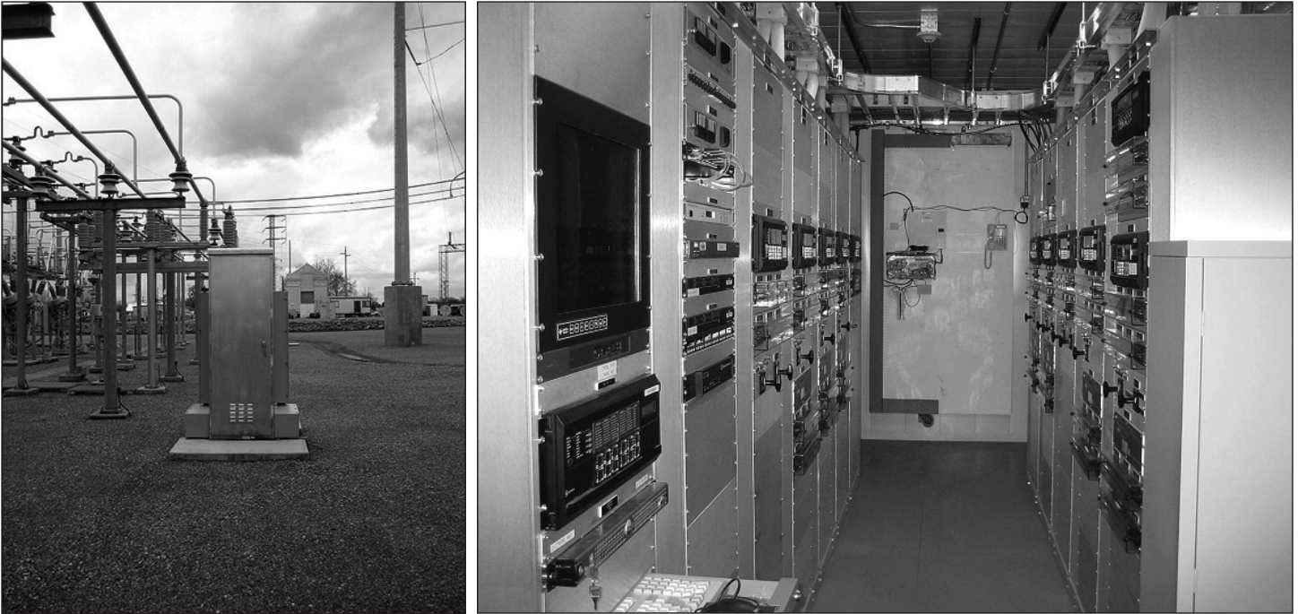
Fig 2. 60 kv bus with outdoor relay cabinet and indoor control building
