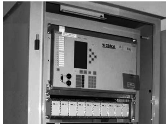
Figure 4. Breaker control IEDs
