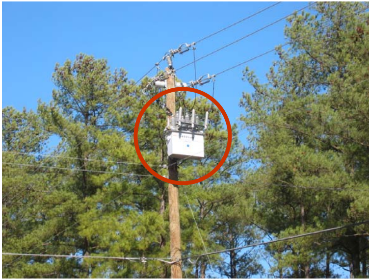
Pole Mount Recloser
