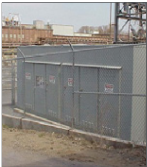
Metal Enclosed Shunt or Filter Bank
