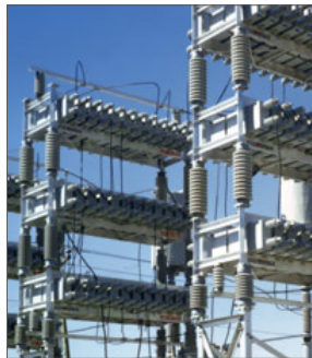
Open Rack Harmonic Filter Bank
