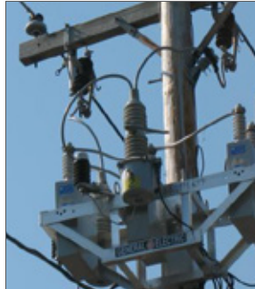
Pole Top Shunt Banks
