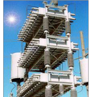
Open Rack Shunt Banks
