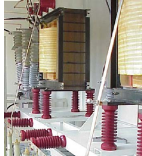
Iron-core harmonic filter reactors used in a 7 MVAR 5th harmonic filter bank. Note extensive use of plated bus for connection of reactors to capacitors.
