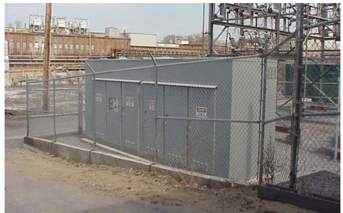
Typical Three-Phase 34.5KV Single-Step 7 MVAR 5th Harmonic Filter Bank.
