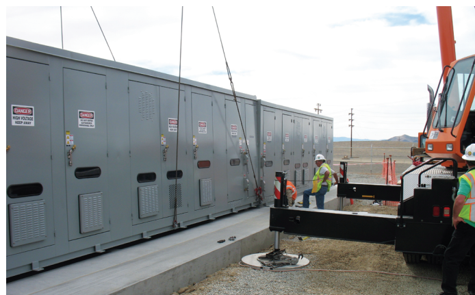
60 MVAR, 38kV, 5-stage 2 section Metal-Enclosed Capacitor Bank being installed at solar plant
