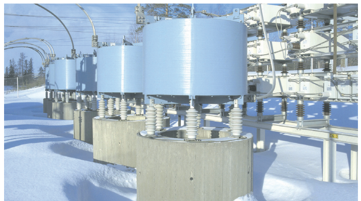
1.4 HV harmonic filter
