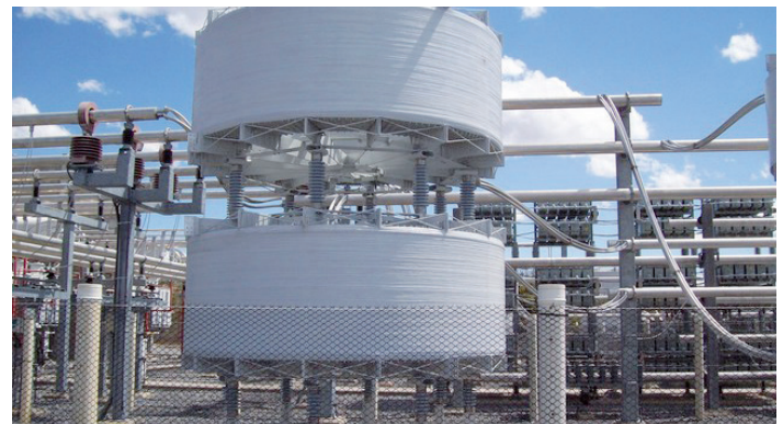
1.5.1 Thyristor Controlled Reactors (TCR)
