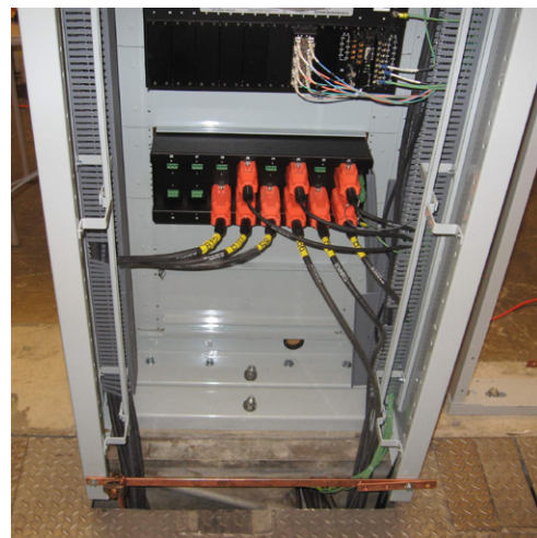
Figure 6: Process bus wiring with fiber optic cables.
