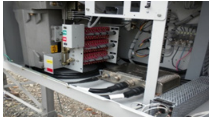
Figure 2: Example of a process interface unit mounted directly inside the equipment cabinet
