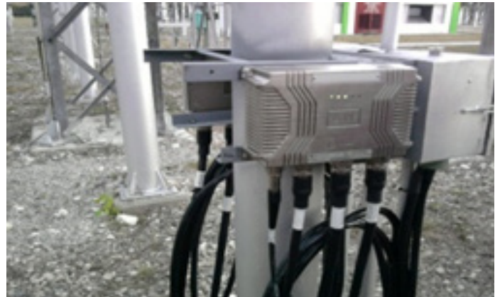
Figure 3: Outdoor mounting of the process interface unit in the switchyard
