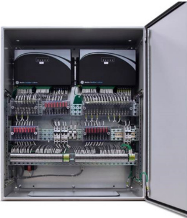
Figure 1: Example of a marshalling cabinet (kiosk) for process interface units
