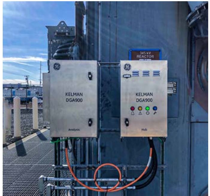
Kelman DGA 900 installed on NYPA transformer
