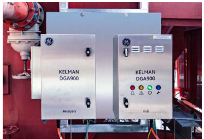
Kelman DGA 900 installed on NYPA transformer
