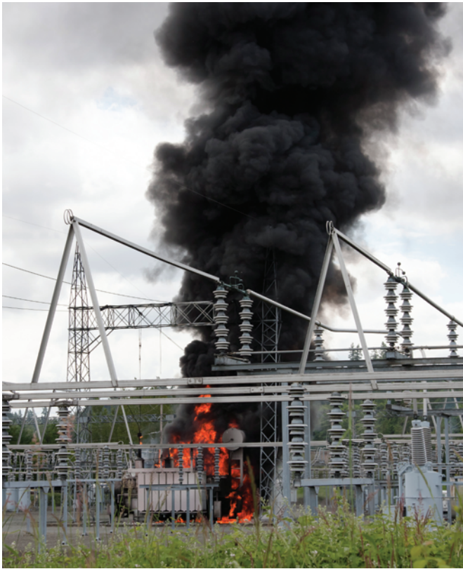
Fig 1: Picture of a sub-station fire resulting from a transformer failure
