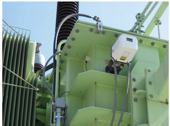
Fig 3: GE's Hydran M2 monitor mounted on a transformer
