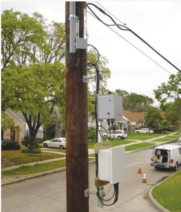
This pole-mounted cell relay and radio in a Houston neighborhood includes (from bottom to top) the weatherproof enclosure for the MDS Mercury 3650 radio, the Itron cell relay weatherproof enclosure and the bottom of the WiMAX antenna.
