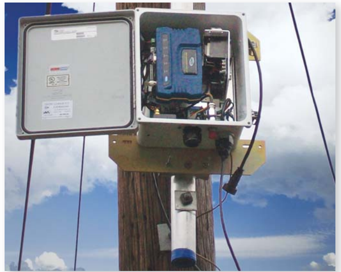
A closeup view of the MDS Mercury 3650 radio in the weatherproof enclosure (with the door open) on the utility pole.
