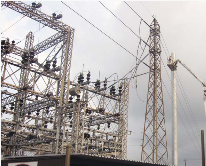
Construction of the takeout point tower (metal pole) at the Dunlavy substation. Before its construction, CenterPoint Energy performed radio signal tests and checked signal strengths to select the remote sites associated with this takeout point.
