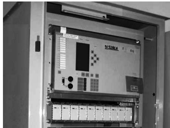
Figure 4. Breaker control IEDs
