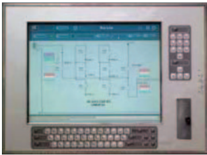
Figure 12. Typical SCADA control monitor
