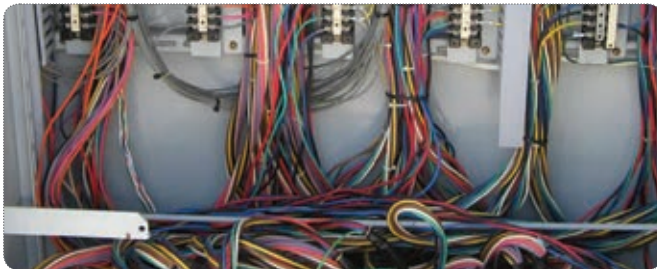
Many connections need to be made in each apparatus in the high voltage equipment switchyard
