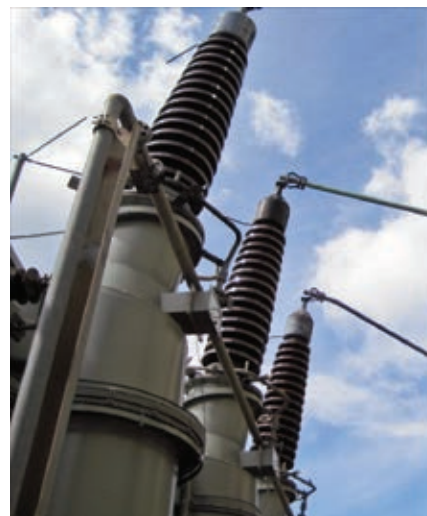
a) Transformer HV Bushings
