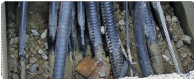
Extensive amounts of copper cables need to be distributed from each switchyard apparatus back to the control house
