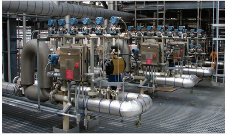
Figure 11: Hydrogen / natural gas blending system.
